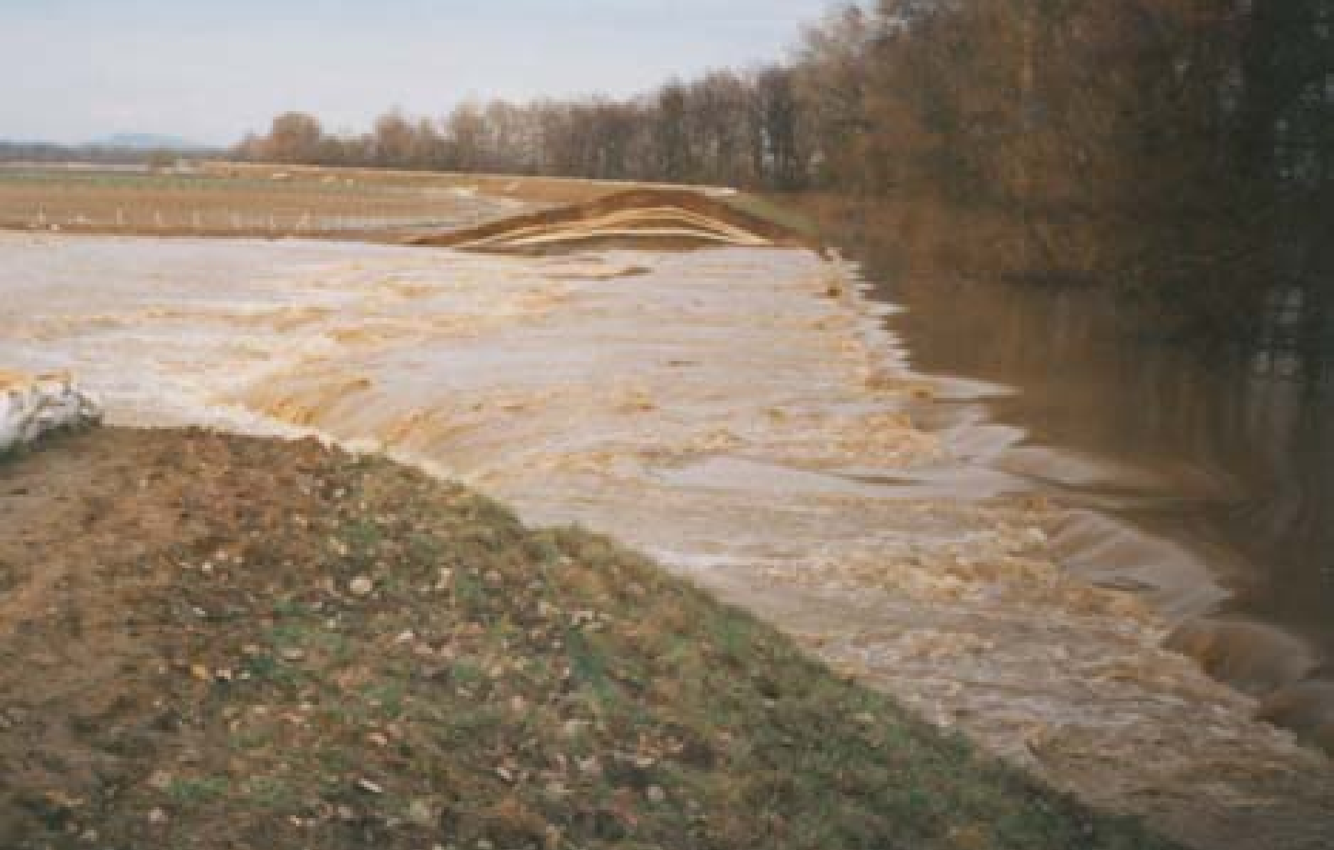
The flood in March 2001 resulted in a dam-break.
